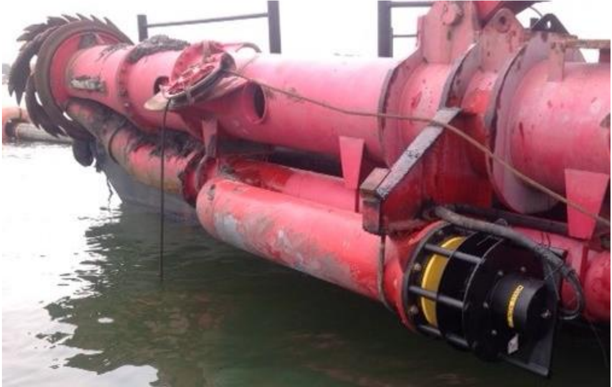
CONVAC LINEAR NEEDLE VALVE ON BYPASS PIPE
